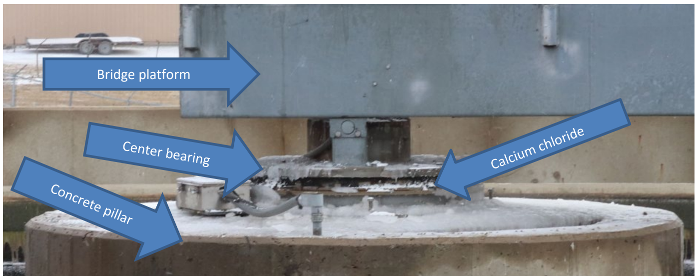
Figure 4 – Calcium chloride on the center bearing (photo credit: Illinois State Police).
