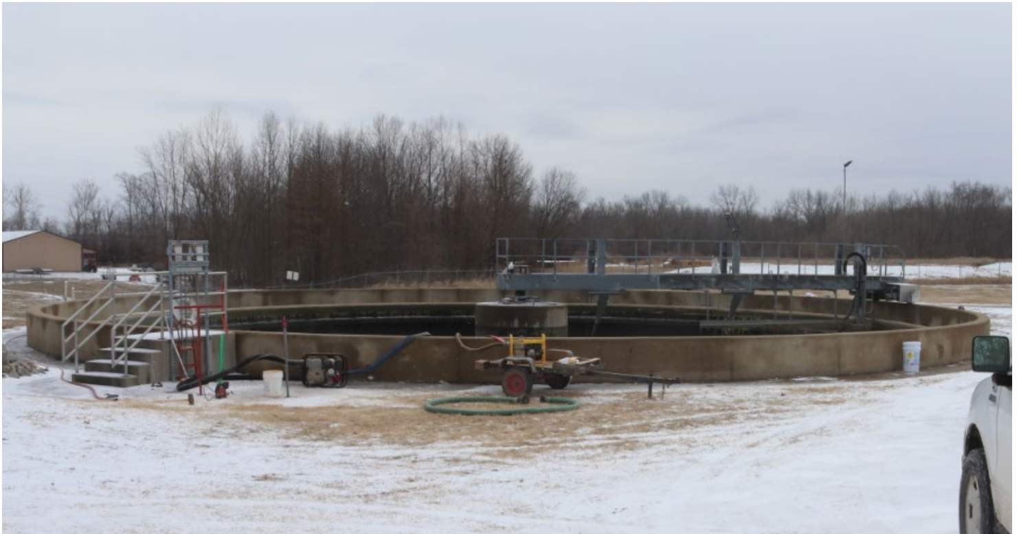
Figure 1 – Clarifier on 2/14/21, post incident (photo credit: Illinois State Police).
