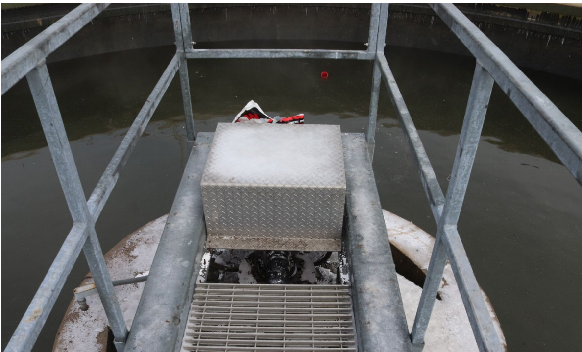
Figure 6 – View from bridge looking at center pillar and bearing. Red object in water is a coffee can presumably used to spread calcium chloride. Note: the clarifier had been drained below the operating level during search and rescue operations (Photo credit: Illinois State Police).
