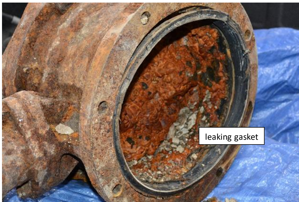
Figure 9 – 12" valve, and gasket that was leaking.
