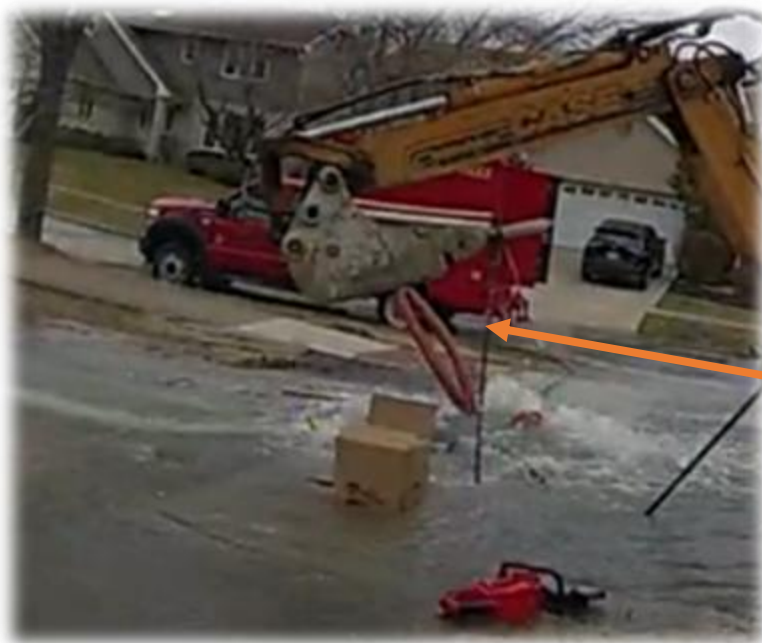
Figure 5 – Still photo of a police officer body camera shows the volume of water that was pouring out of the vault. Note the chain attached to the backhoe going into the manhole.
