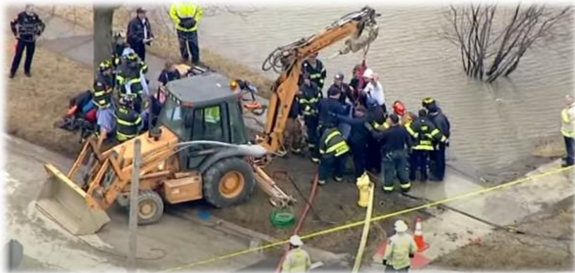
Figure 7 – Aerial view of incident scene as worker #1 is removed from the vault. (Photo credit: ABC 7 News Chicago)
