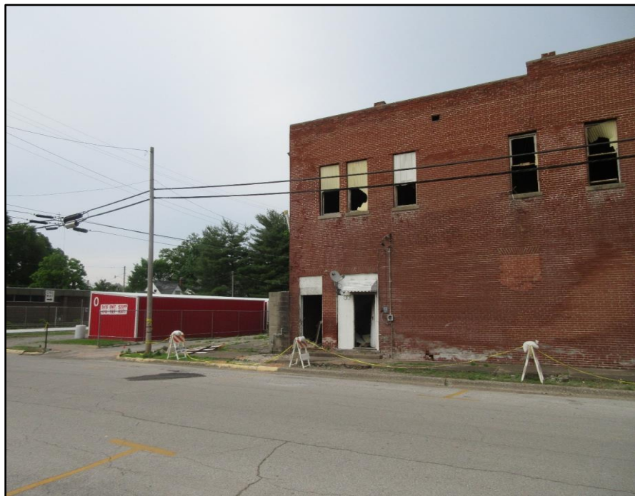
Side Bravo north and south doors, shown left to right. Engine 201 firefighters placed a ground ladder to the completely cleared window on the 2 nd floor. NIOSH Photo
