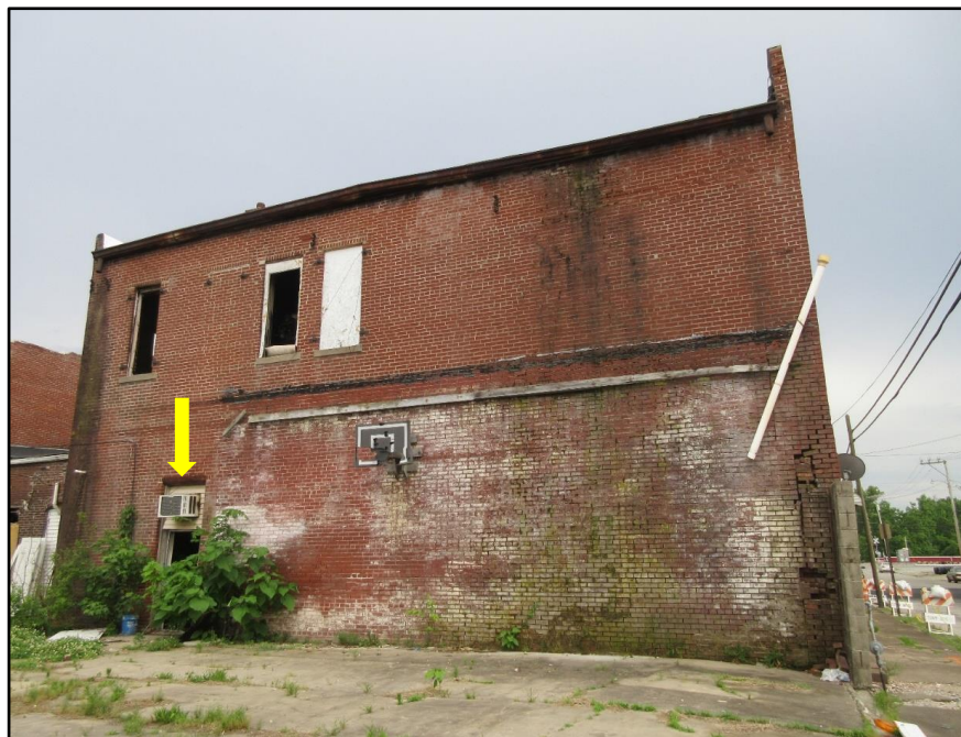
Side Charlie door with A/C unit over top of it. The stairwell landing to 2nd floor that collapsed is just above door and A/C unit inside the wall. Photo by NIOSH
