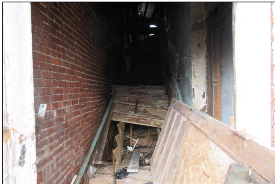
The stairwell against Side Charlie where the lieutenant and firefighter made entry to 2 nd floor. The lieutenant was rescued by RIT underneath of the stairwell.
